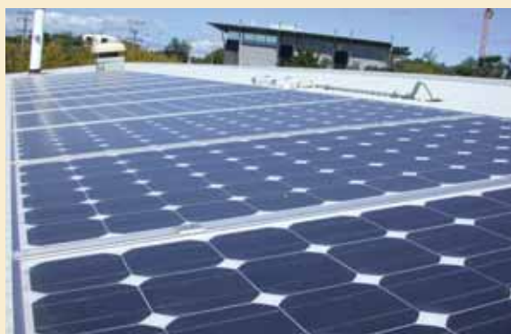
12 PV panels mounted on Science Block, Westlake Girls High School, Auckland
